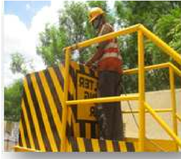
Air cleaner cleaning hopper
